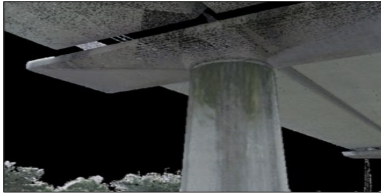
Figure 7. Moss on Pier 27 initial data
